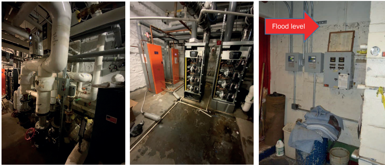
Figure 7. Damage to equipment in flooded basements
