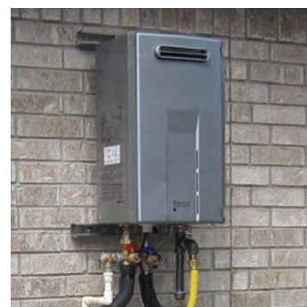
▲ Tankless water heater affixed to a building servicing the insured property.
