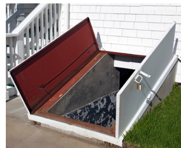
▲ Exterior egress in a basement is not covered.
