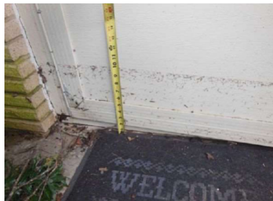
▲ Example of a good photograph: clear picture of the waterline with measurement.
