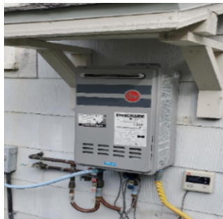
▲ A gas-fired flash water heater affixed to the building's exterior siding, making it part of the building and therefore covered.
