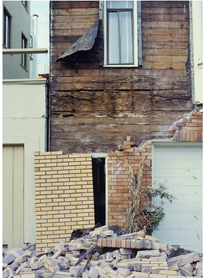
Brick masonry veneer fallen off of home exterior.
