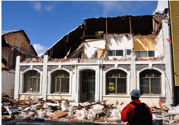
Photo of damage to masonry building in Christchurch. COURTESY OF FRED TURNER, AVAILABLE AT WWW.EERI.ORG, LAST ACCESSED 8/3/19
